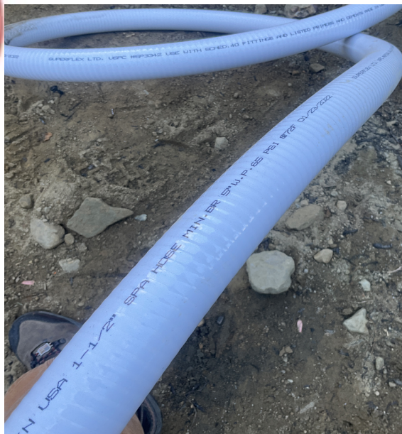
This piping is often bought, but it is not listed in the pool/spa code.
